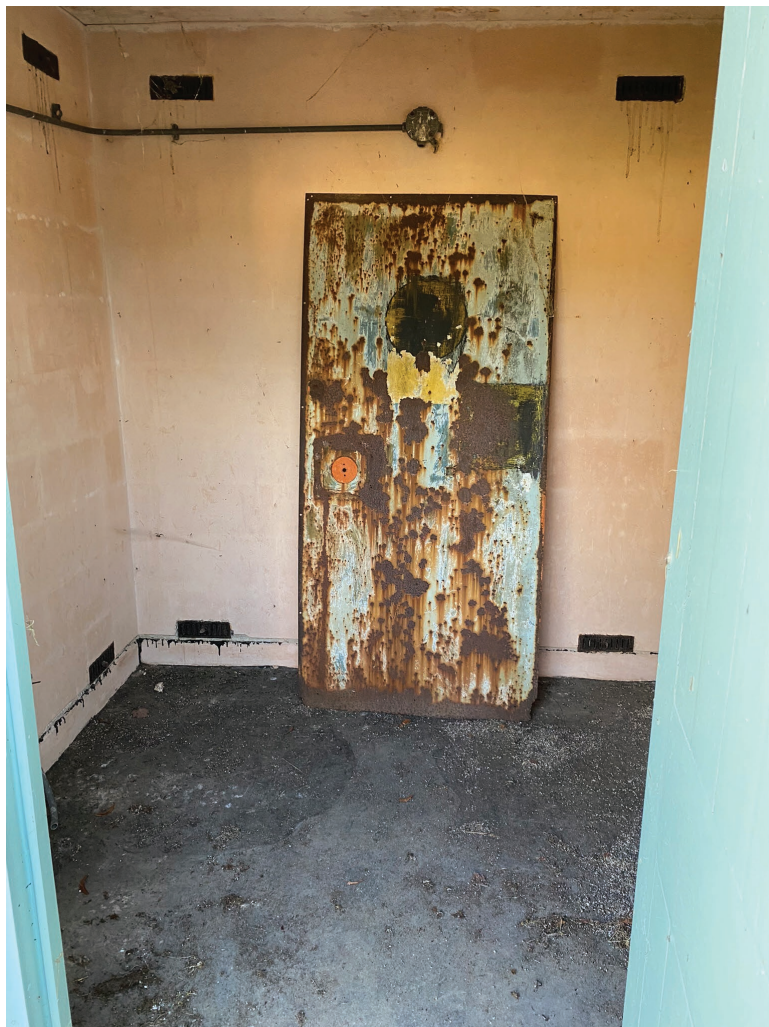
Figure 14.2 Original iron doors inside the hutch at Gorse Industrial Estate (formerly RAF Barnham)
